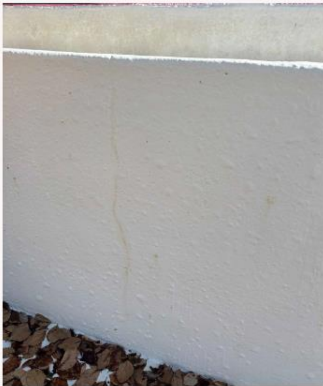
Figure 2: Stress fractures along pool basin wall.
