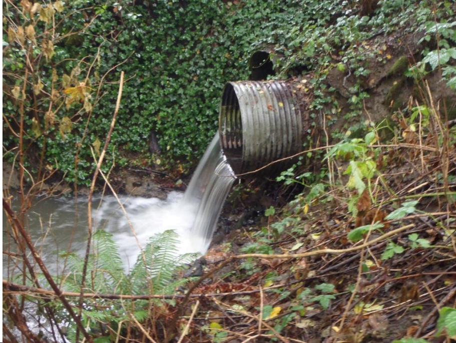
Photo 5. View north of the approx. 1 m drop from the culvert outlet under 10th St. East, downstream of the subject property, acting as a complete barrier to anadromous fish migration.
