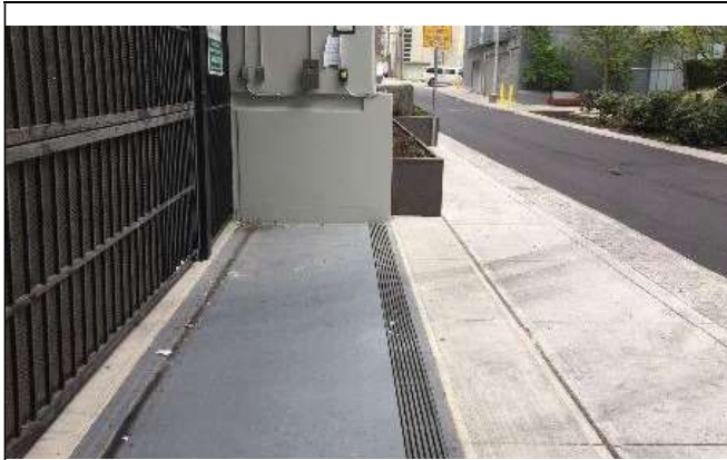
FloodBreak barrier (not activated) at Mountain Equipment Company, Vancouver. (Credit: FloodBreak).
