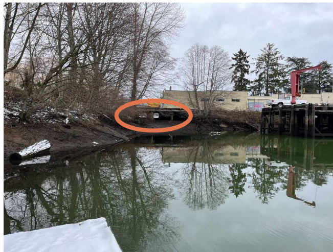
Figure 6-33: View of Lewis Park culverts from the South from Courtenay Slough. (Credit: Ebbwater, 27 Feb 2023).
