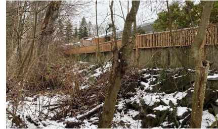
Figure 6-17: Canterbury Lane Dike, with setback concrete wall, riprap toe protection and fencing, with residential complex immediately behind structure. (Credit: Water Street Eng., 27 Feb 2023)
