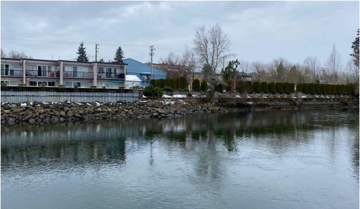
Photo 1: Anderton Dike transitions from concrete wall at northern upstream side (right side of photo) to sheet pile wall with a concrete cap (left side of photo).
