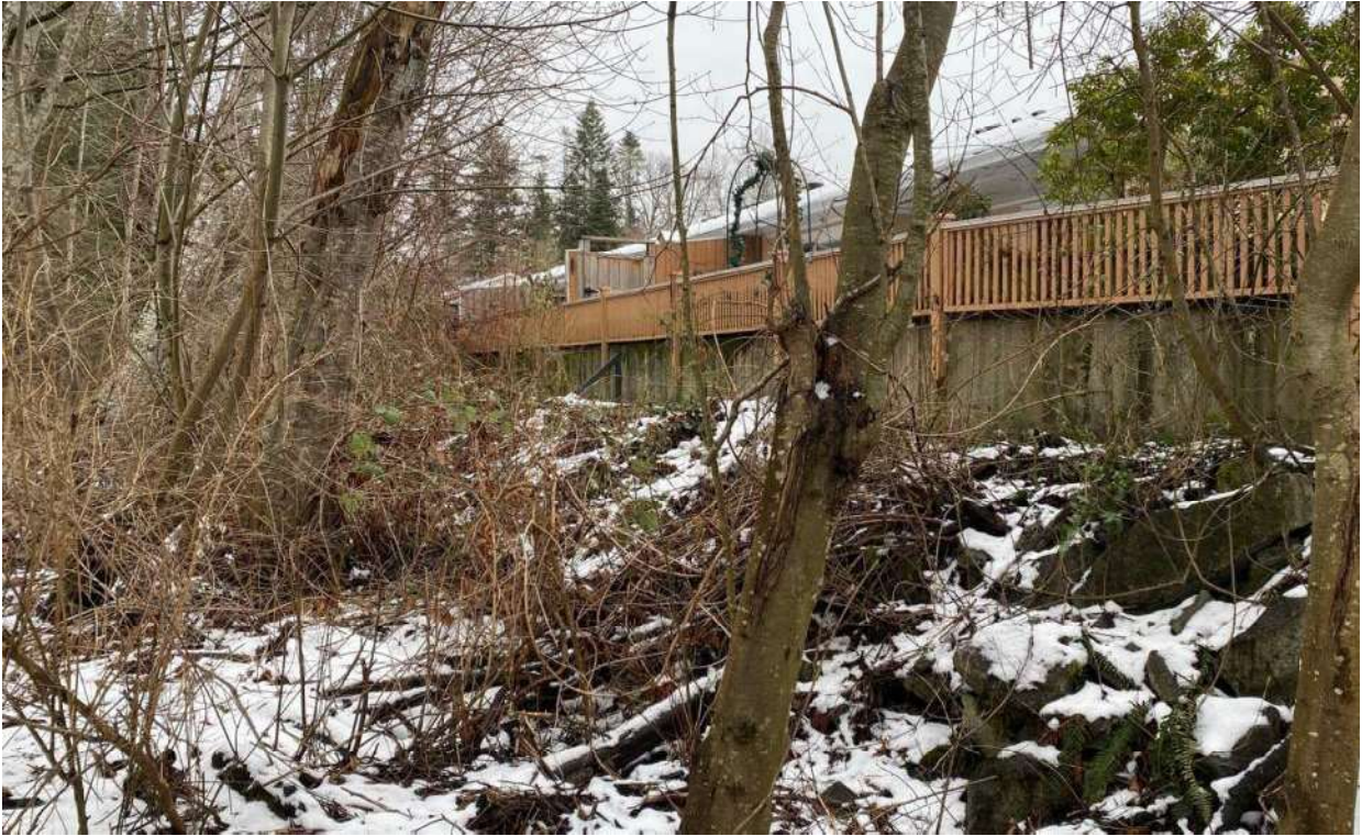
Photo 18: Canterbury Lane Dike with setback concrete wall, riprap toe protection, and fencing visible.
