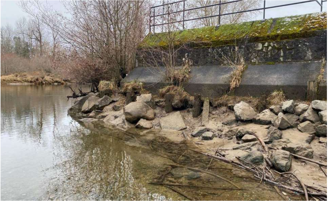
Photo 10: Riprap placed around toe of the Lewis Park Dike at the bend in the Courtenay River.
