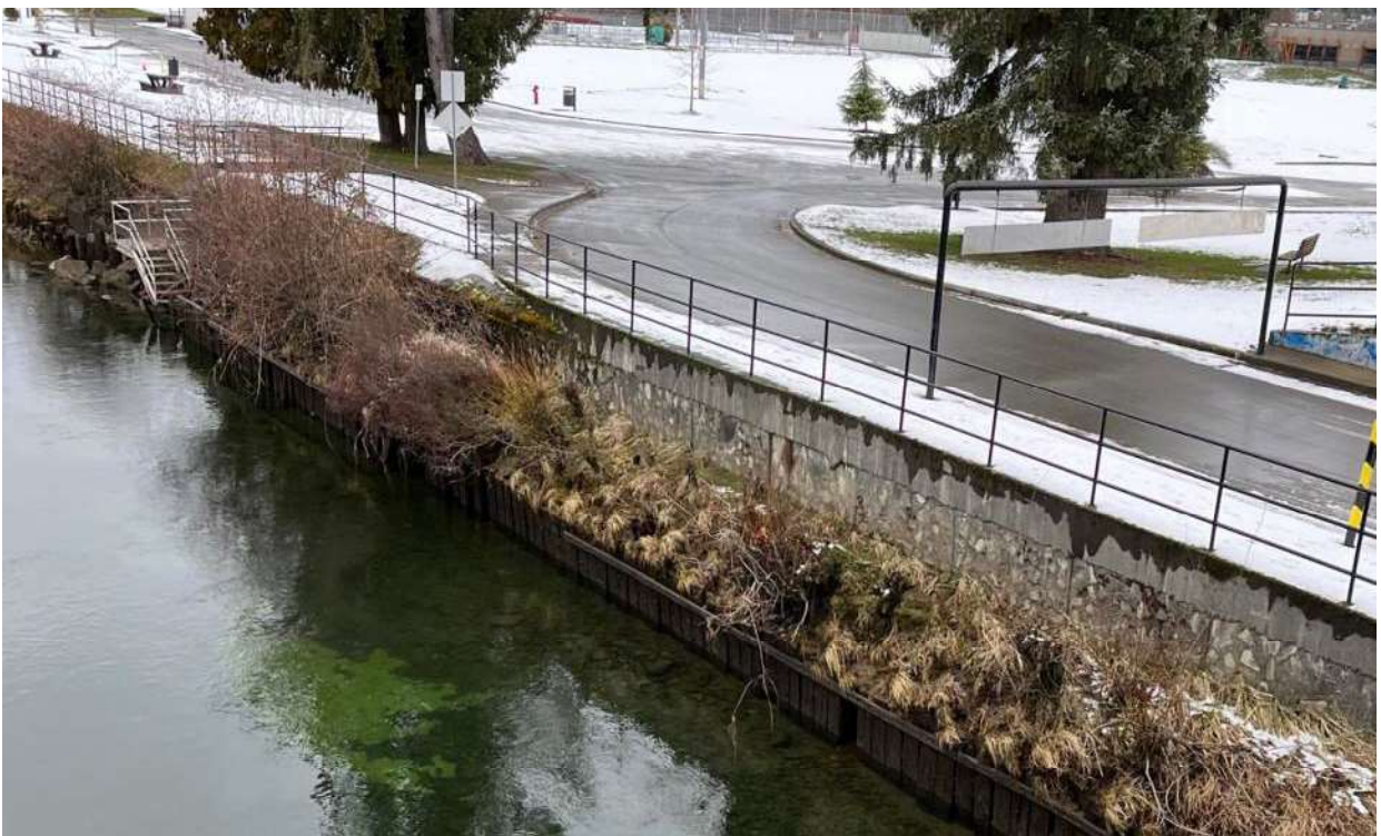
Photo 11: Riprap placed around stairs and foundation of the Lewis Park Dike at the upstream (southern) section.
