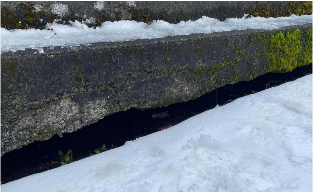
Photo 4: Gap underneath the concrete cap of the sheet pile wall of the Anderton Dike on the land side.
