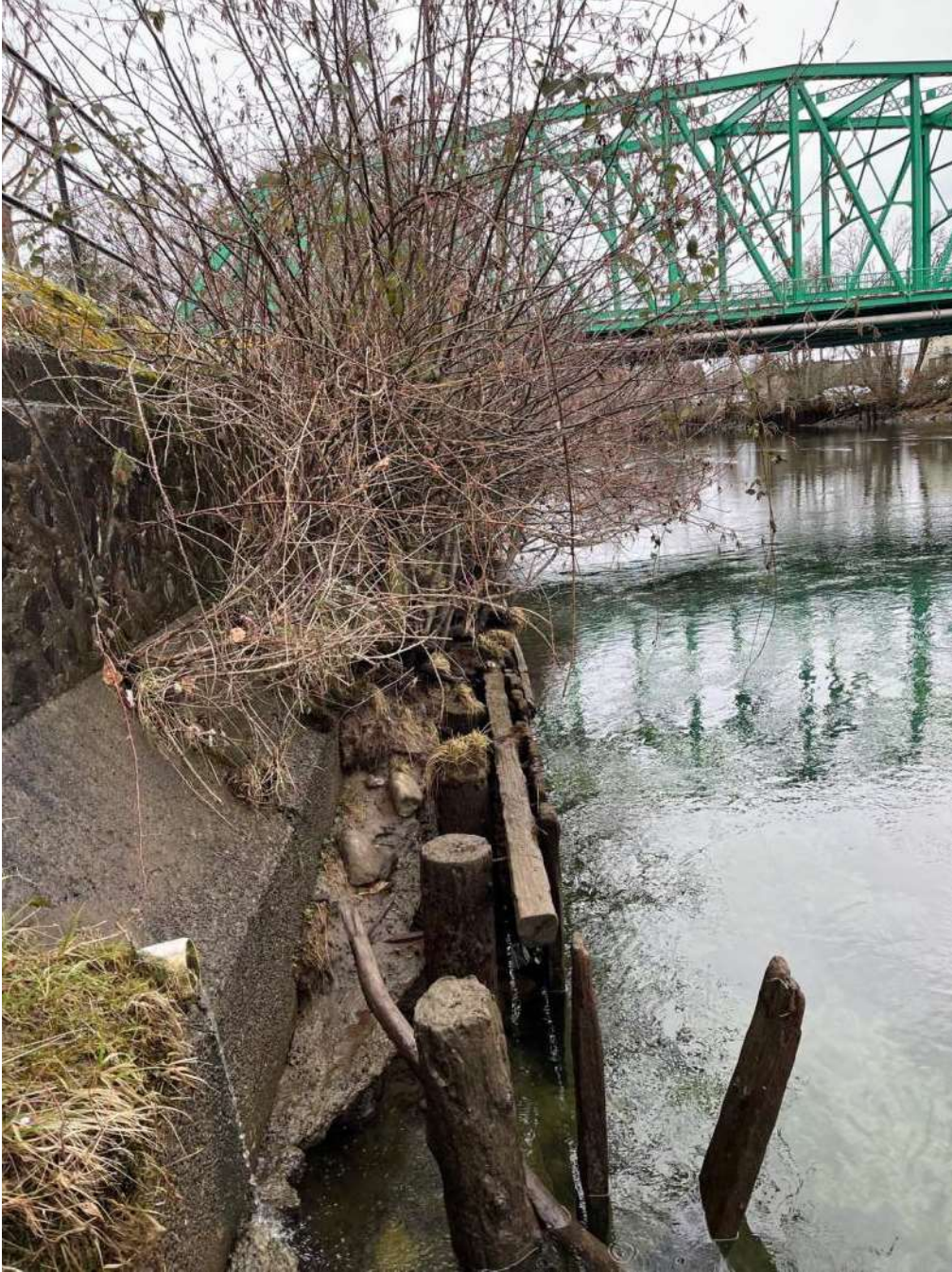
Photo 8: Remnants of old log wall in front of concrete structure. Stormwater outfall discharging onto toe.
