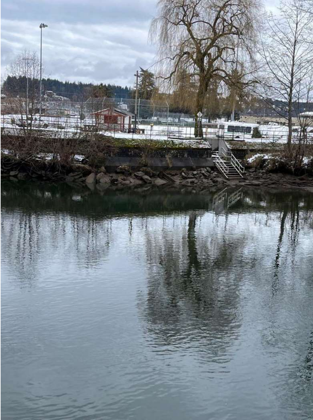
Photo 9: Large riprap placed around stairs and foundation of the Lewis Park Dike.
