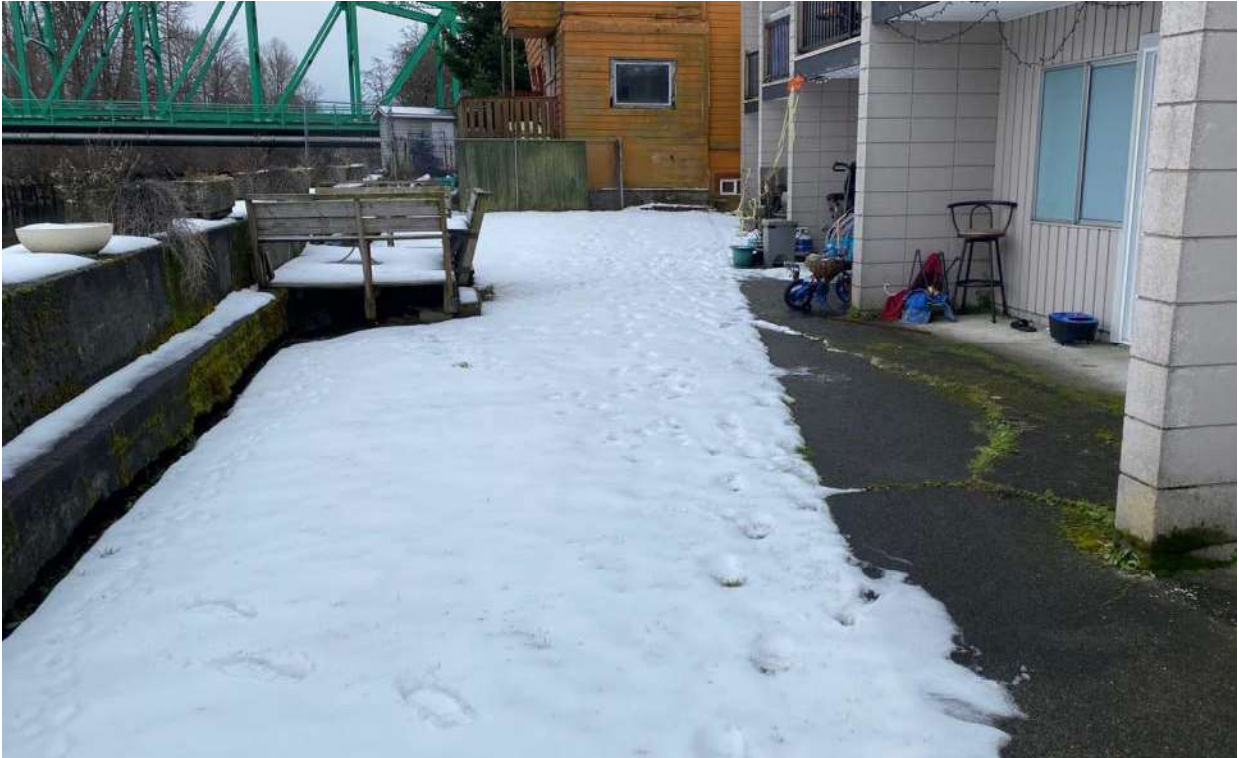
Photo 3: Ground cracking observed behind the Anderton Dike wall in the backyard of the apartment buildings.
