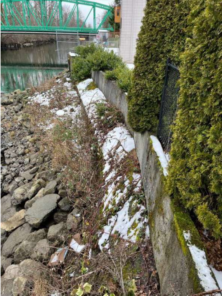
Photo 5: Vegetation observed within the Anderton concrete wall and riprap.
