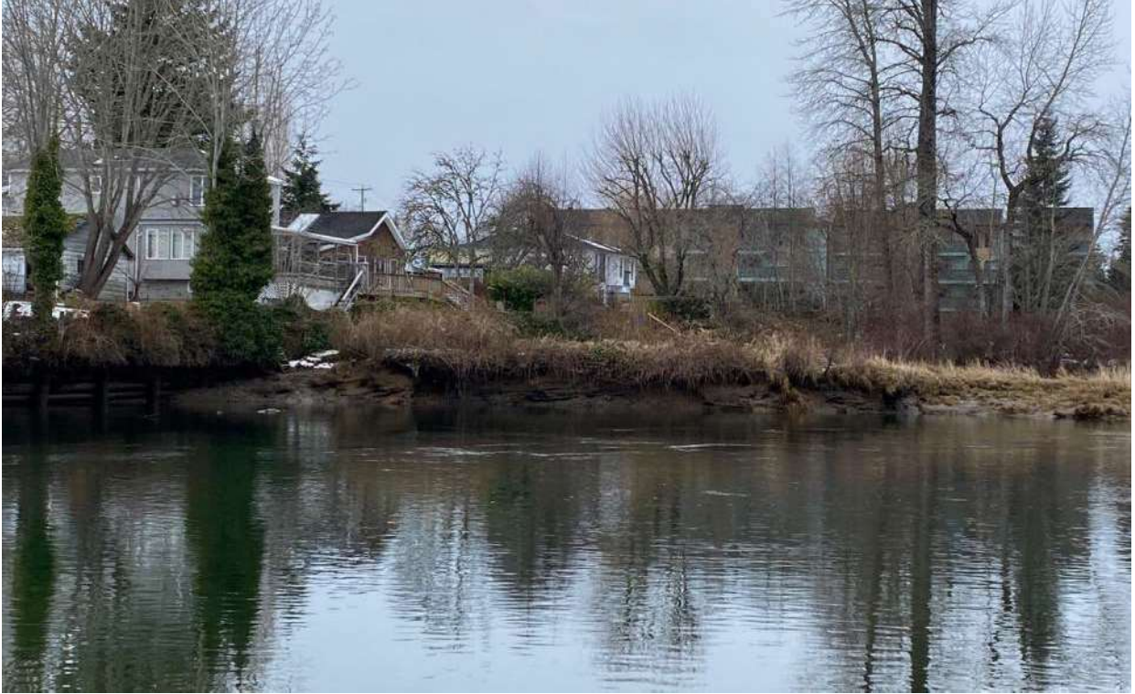
Photo 6: Ongoing erosion at the bend upstream of the Anderton Dike at approximately 1 st Street and Anderton Avenue.
