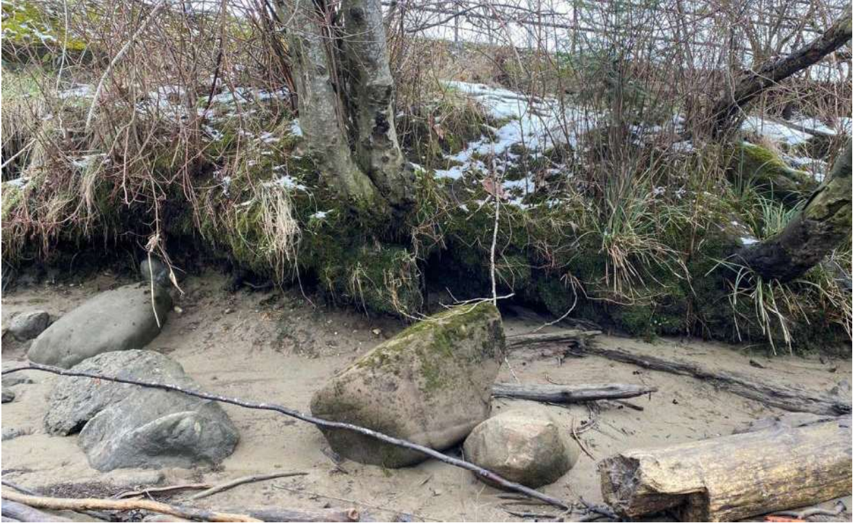
Photo 12: Localized erosion and undermining of material at the Lewis Park Dike at the river bend at approximately 1 st Street and Anderton Avenue.
