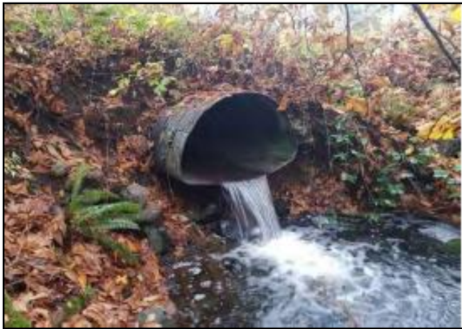
Perched culvert, along Piercy Creek
